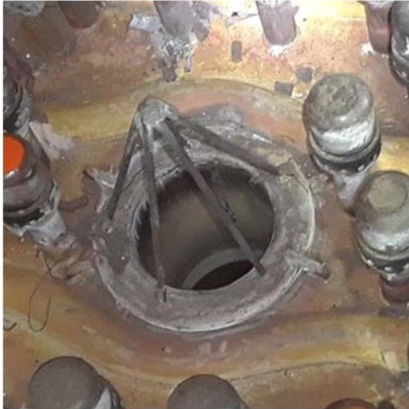
Pic 2: Close up of "Witches Hat Strainer" on one of the four ash drain pipes
