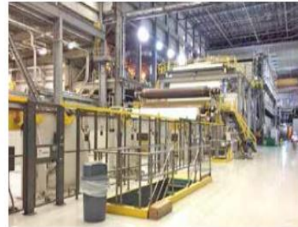
Perimeter guarding around in-running nip points.
