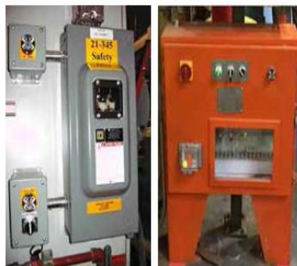
Arc flash mitigation controls for local disconnect switches. Electrical panel with both phase indicator lights and viewing window to aid in verification of zero electrical energy.
