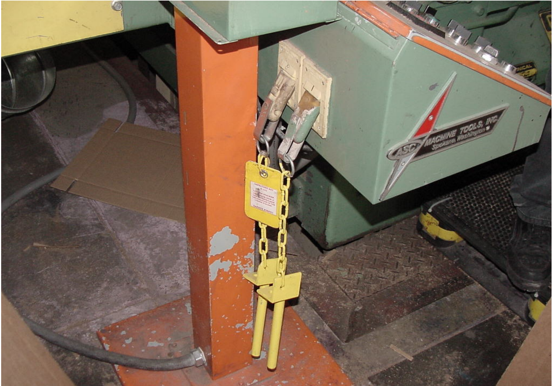
Load Former Disconnects & Safety Pins
